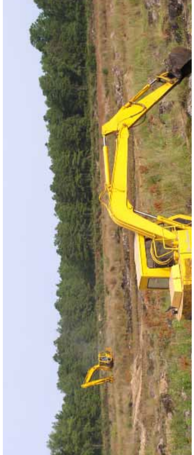
Earth movers dig up old cranberry bogs to create hummocks and depressions for wetlands restoration in the Franklin Parker Preserve, where New Jersey Conservation Foundation is restoring a highly modified agricultural area to wetlands.
